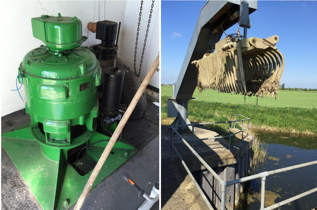
Figure 1 Pump and Weed Screen
