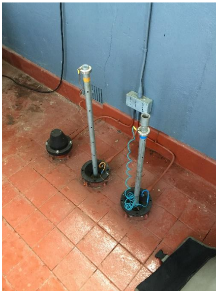
Figure 3 Capacitance Level Switches used to automatically start/stop pumps
