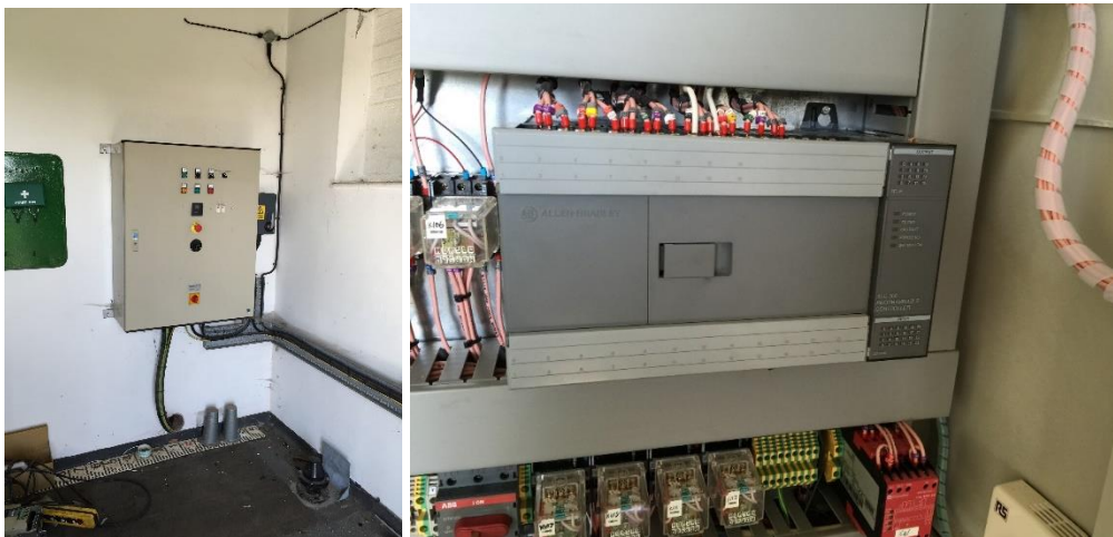
Figure 5 Weed Screen Control Panel
